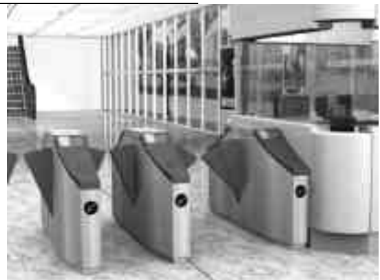
Automatic fare gates
